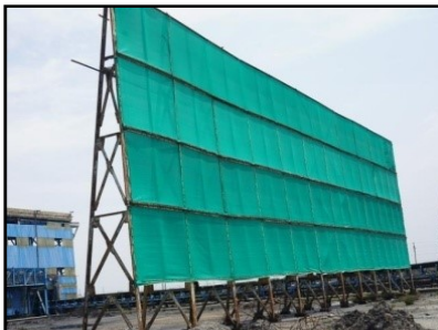
Fig 7: Wind barrier for coal stock yard at NTECL
