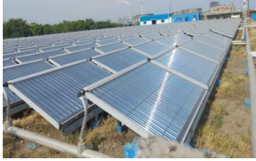
Fig 1: Solar Desalination Plant installed at NTECL
